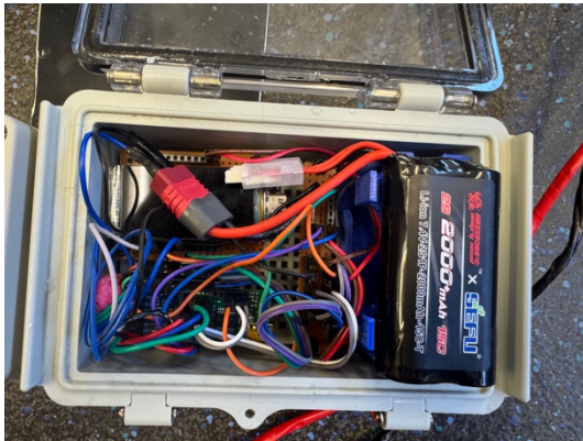
Figure 25 Final Electronics Box Internals
