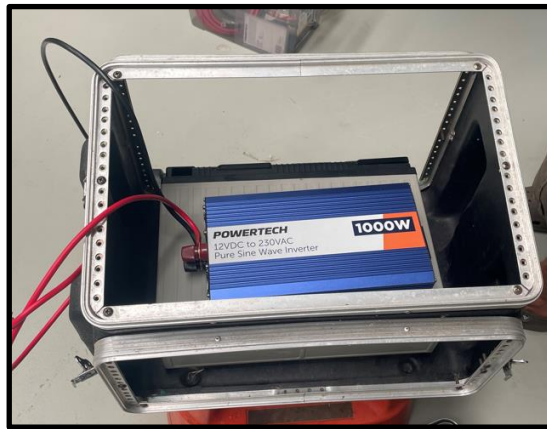
Figure 9: Donated Components: Casing, Battery & Inverter
