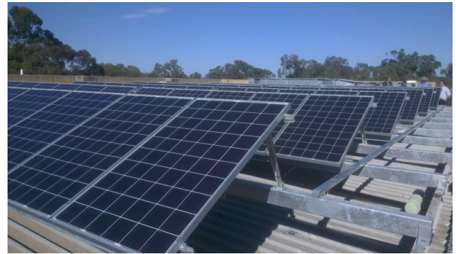
Fig. 1. A 20kW solar system on the Human Movement building of UWA, Western Australia
