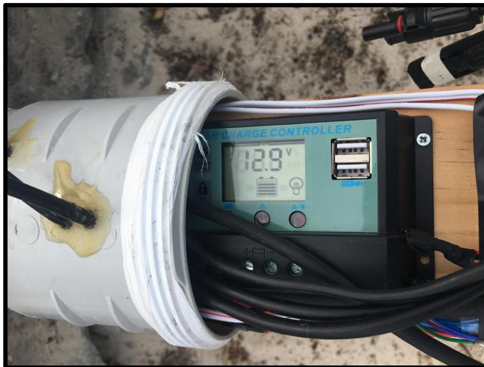
Figure 23: Post Test Battery Check
