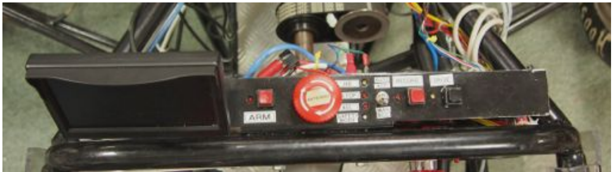
Figure 33: Control panel for safety system and car based interface.
