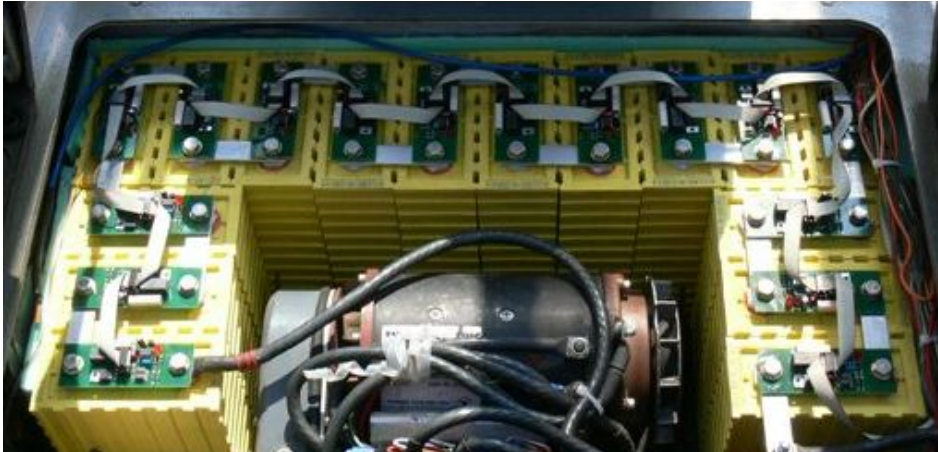
Figure 3.7: A real-world distributed BMS setup. Image courtesy of GK Anlagetechnik.
