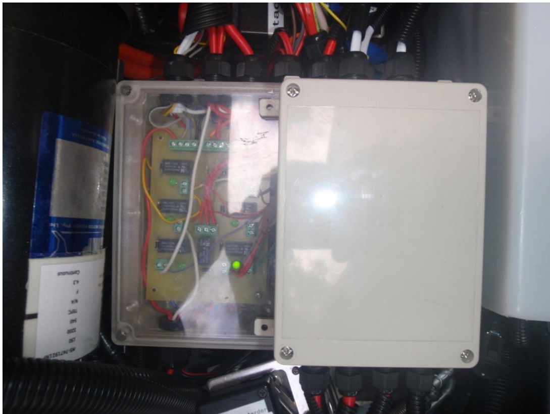
Figure 23: Photo of the Installed 12V distribution and Relay Box
