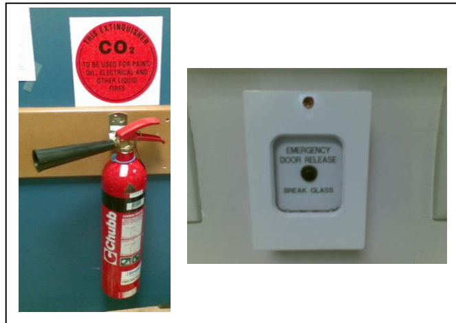
Figure 5.3 Fire extinguisher and emergency door release button mounted in G50 Laboratory
